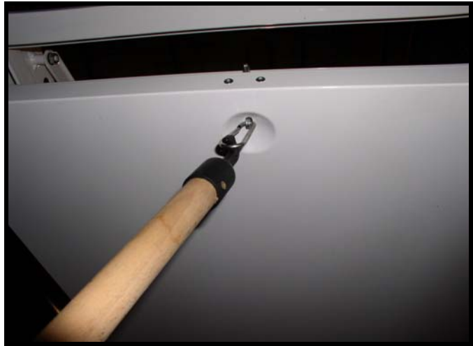
Pull door open using pole and hook.
